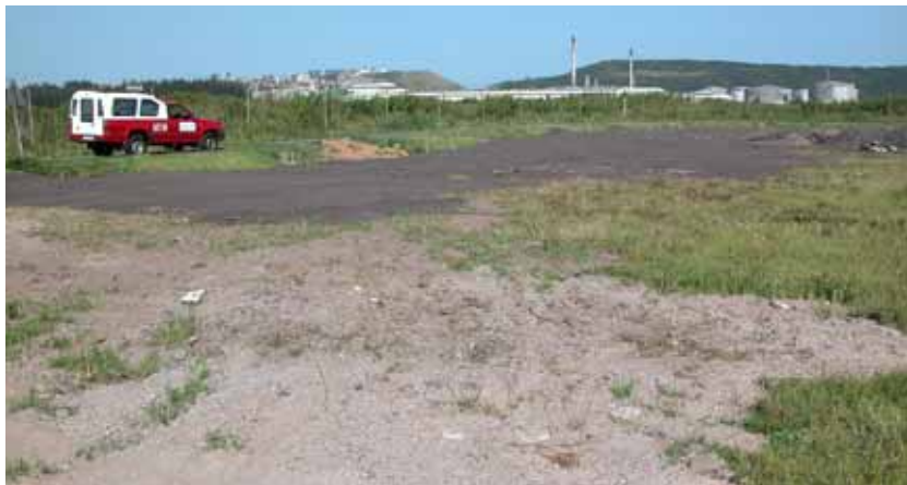
Figure 6. An area where standing water collected has now been filled in with rubble and covered with soil.
